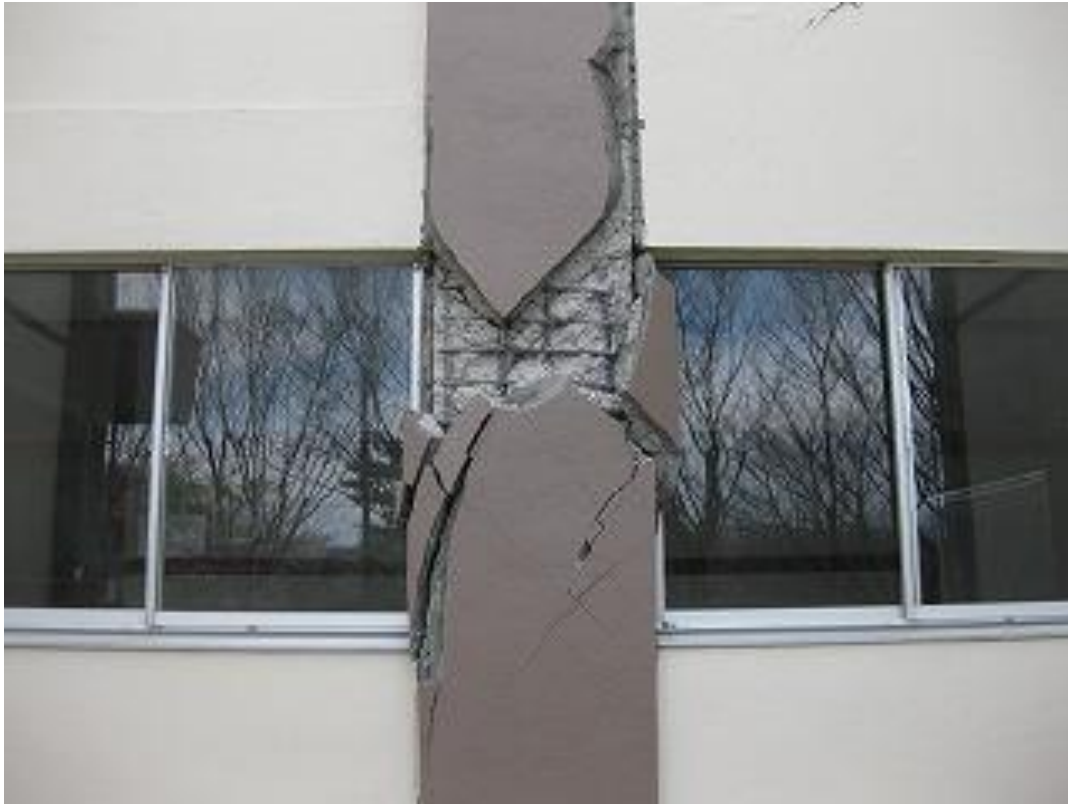
Short column failed in shear
