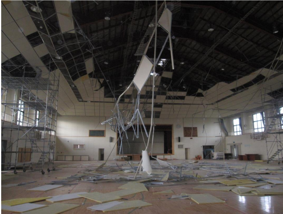
Large parts of the ceiling fell down (3/11, and also in 4/7)
